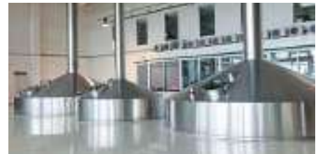
Brewery production equipment
