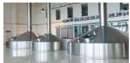
Brewery production equipment
