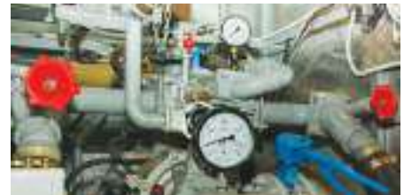
Pump and valve control
