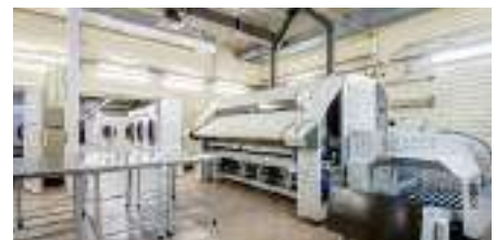
Automated laundry system
