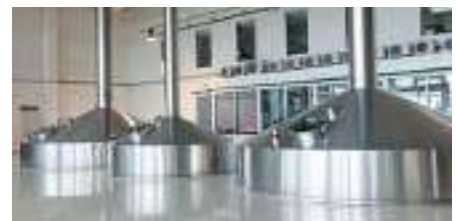
Brewery production equipment
